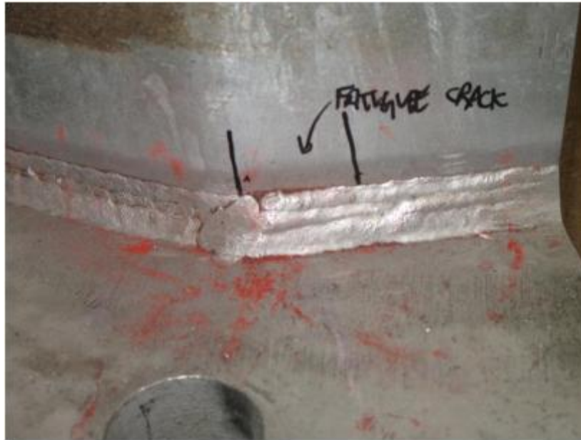
Figure 3.1 Fatigue Crack Observed Using Magnetic Particle Testing
